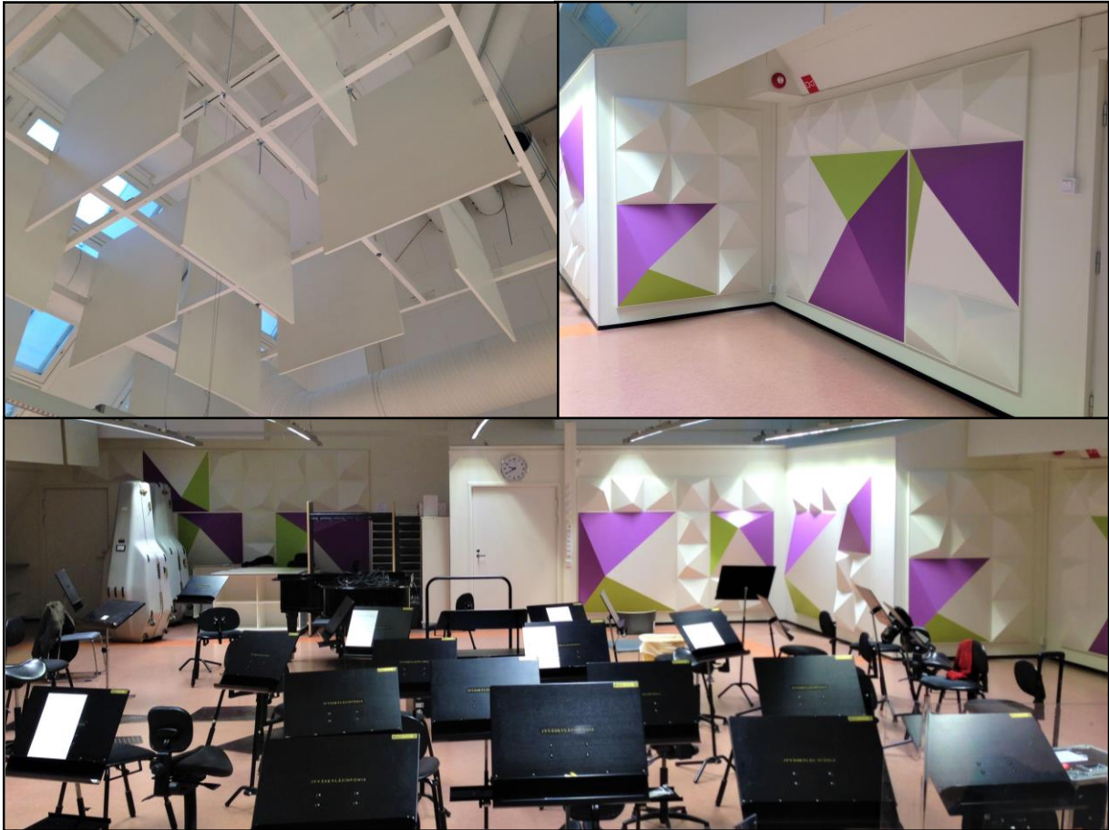
Figure 4: The rehearsal hall after the renovations. The newly mounted ceiling (top left) and wall diffusers (top right) can be seen in the image.
